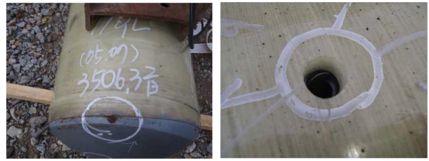
Fig. 15 Photograph of external defect (test 3)
